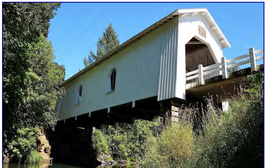
The Hoffman Bridge near the town of Scio was built by hand in 1936, and is still carrying vehicles today.
